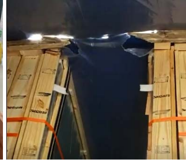
Broken Wood Support
